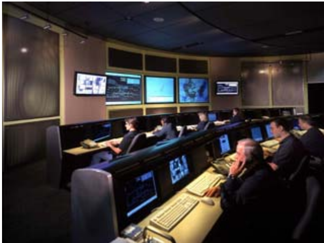
Data Center where Maintenance Connection servers reside
